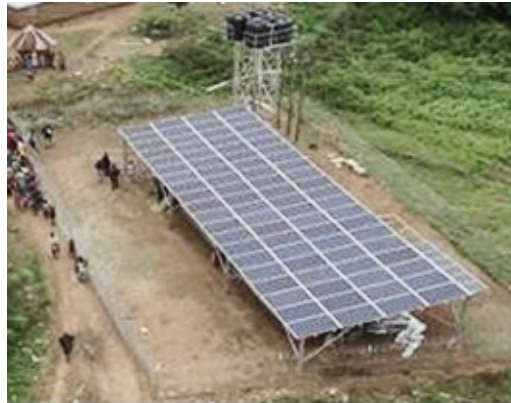
Solar Power Generation
